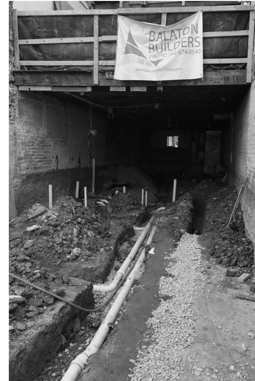
In order to create 9ft high ceilings and allow more natural light into the lower units, the builder had to dig out below the foundation of the building.
