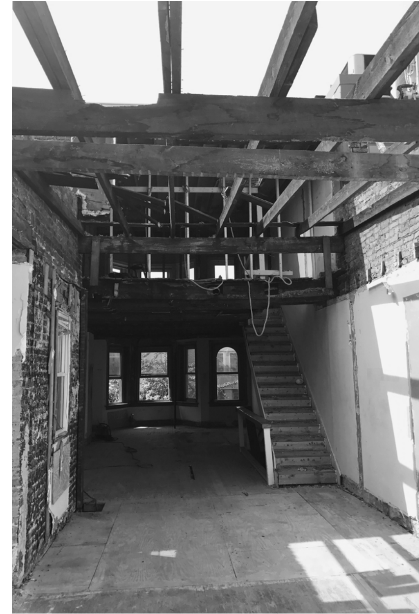
The developer hired the nonprofit corporation, Second Chance, to “deconstruct” the majority of the old building structure for future repurposing.
